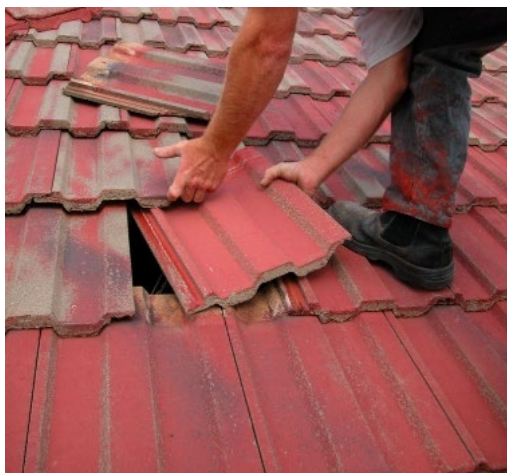
REPLACE BROKEN TILES
