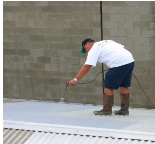
FIRST COAT – ACRYLOC PRIMERBOND METAL & GALV PRIMER. (ROOF RESTORE ON OLD C/BOND)
