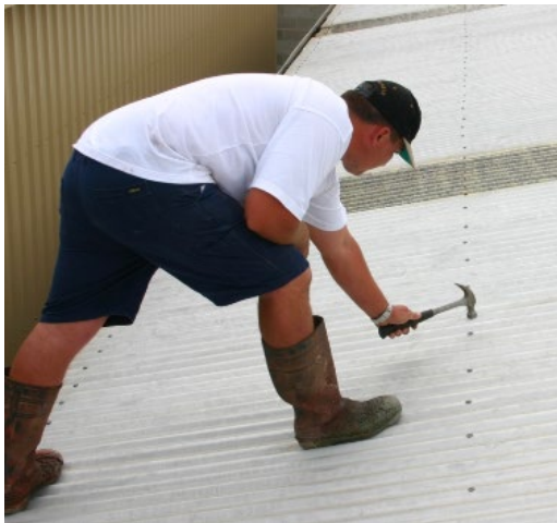
REPLACE DAMAGED SHEETS, FIX LOOSE NAILS OR SCREWS
